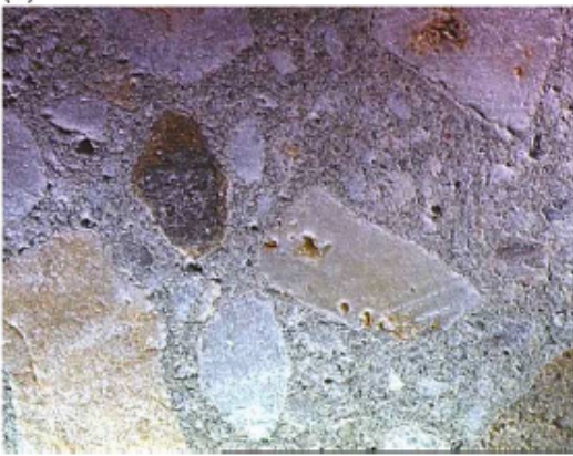
Pit formation due to cavitation
